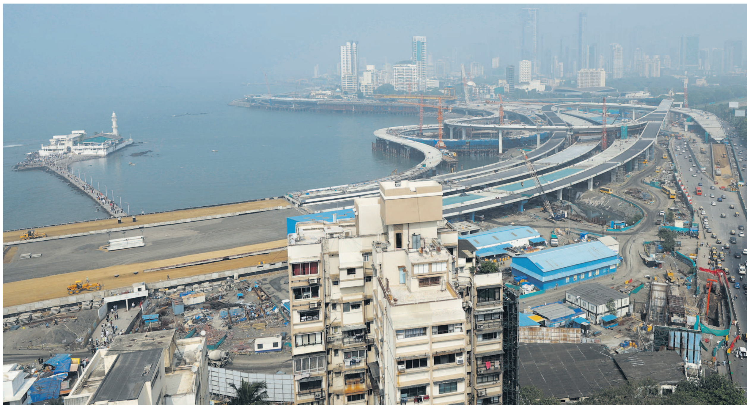
A general view of residential buildings amid the coastal road construction work in Mumbai on 1 December. The Mumbai metropolitan region (MMR) currently has 592,650 residential units under construction
