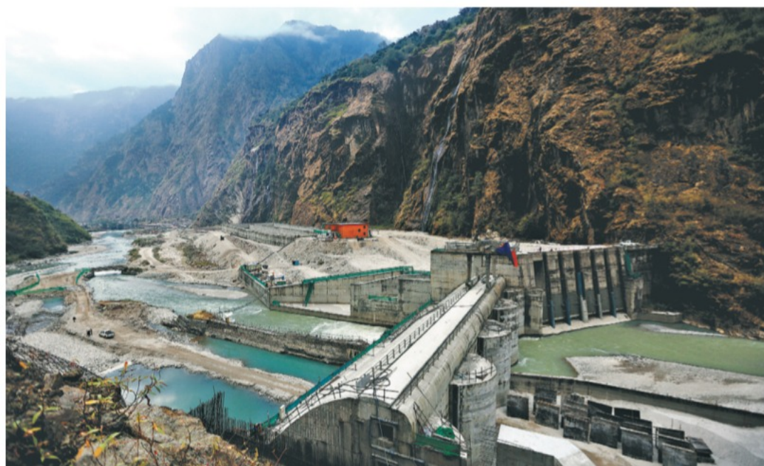
The 456MW Upper Tamakoshi in Dolakha currently stands as Nepal's biggest hydroelectricity project.
